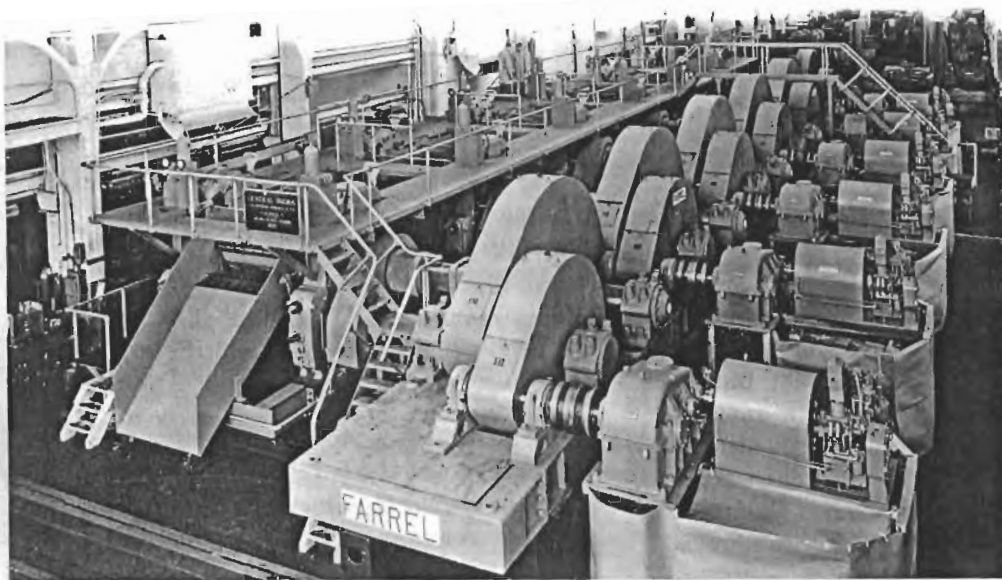
FIGURE 26 — Tandem sugar mill consisting of six three-roll mills, each with its own turbine drive. Grinding capacity is 3000 tons of cane per day. Enclosed reduction gears are closed herringbone type
